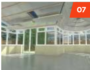
3 layers of high performance insulation (between and over rafters, and insulated plasterboard), is installed.
