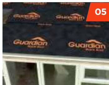
Breathable waterproof membrane is laid over the ply-wood and secured in place.
