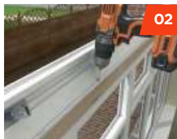
Timber packer and structural ring-beam are sealed and secured to the top of the window frames.
