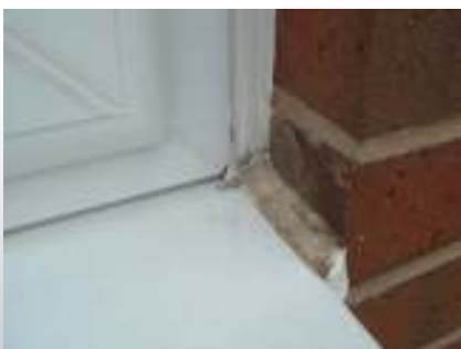
Unsightly & non energy efficient window installation
